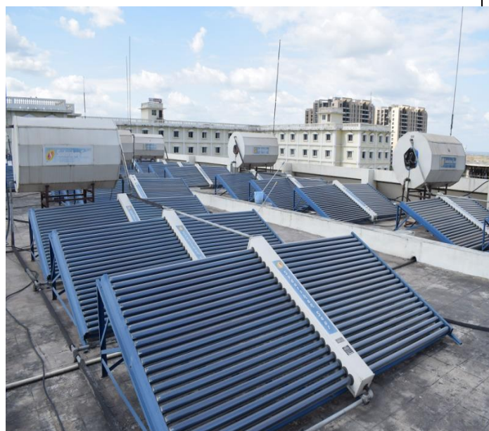
Photo No. 13 Solar Water Heating for Hostels
